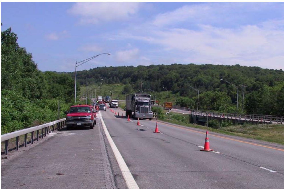
Photo 1. The site of the fatal incident where the southbound driving lane was closed to the traffic and the work zone was demarcated with orange traffic cones.
