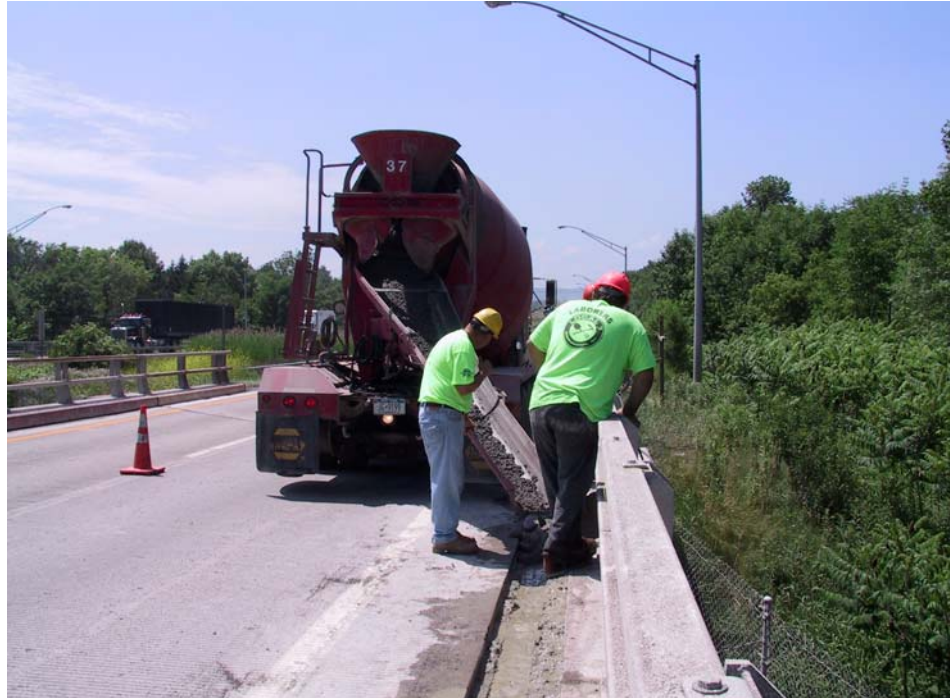
Photo 2. Paving company employees working at the rear end of the cement truck. (Photo was taken the day after work resumed, one month after the fatal incident. The cement truck and the workers pictured are in the same position as the victims at the time of the fatal incident.)
