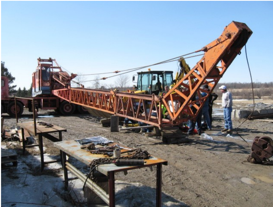
Photo 3. The boom assembly buckled at two locations: between the tip and extension II and between extensions I and II. The victim was crushed by extension II. Blocking under the boom was placed after the incident. (Photo courtesy of OHSa)
