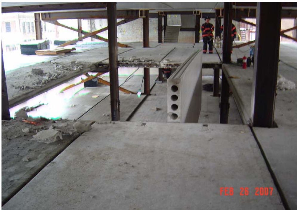
Photo 4. A 4th floor slab adjacent to the collapsed zone was pushed to a vertical position and wedged between the steel beams. (Photo courtesy of OSHA)
