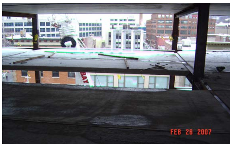
Photo 2. The initial collapsing zone on 6th floor. (Photo courtesy of OSHA)
