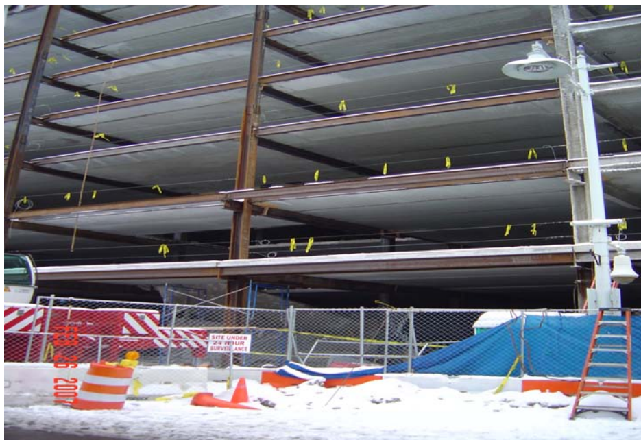
Photo 1. The north side of the precast concrete building. (Photo courtesy of OSHA)
