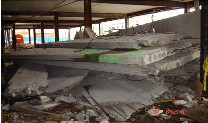
Photo 3. The domino effect started by the failed slab on the 6th floor crashing through the five floors below and caused the collapse of five more slabs to the ground level. (Photo courtesy of OSHA)
